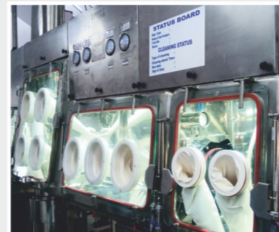
ANFD Discharge Isolator
